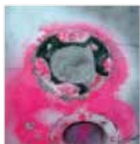
Concrete filled sleeves
