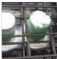
Cracked and broken Sleeves
